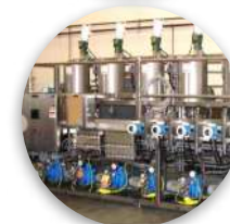
AC & DC Servo Systems, Drives, Instrumentation Control Valve and PLC integration
