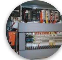
Electrical Control Panels
