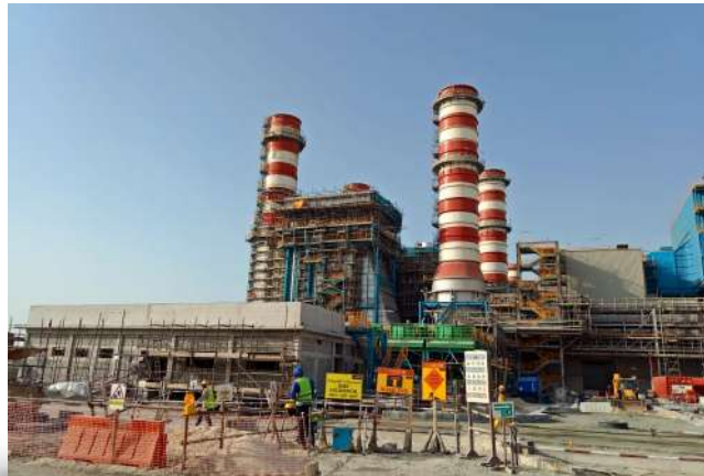
Jamex Power Plant, Jebel Ali Free Zone, UAE
