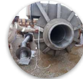
Cyclone Converter Installation
